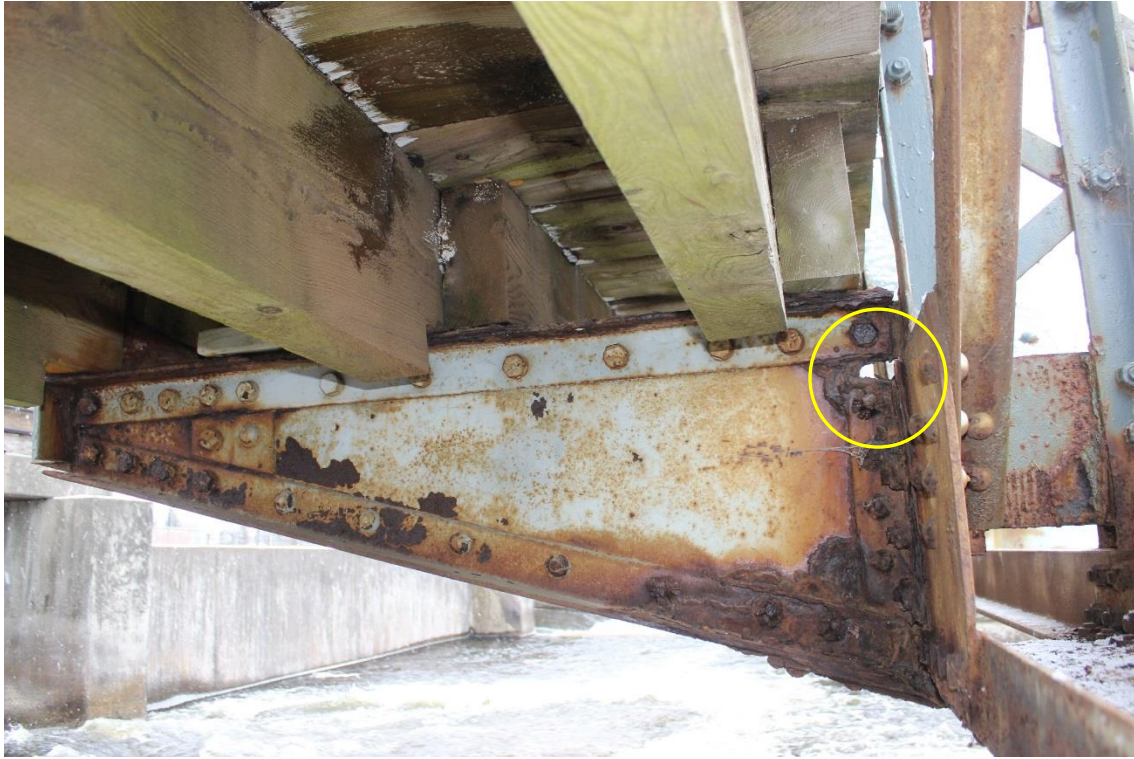
Image 9. Minor perforation sidewalk outrigger panel point 4 east truss
