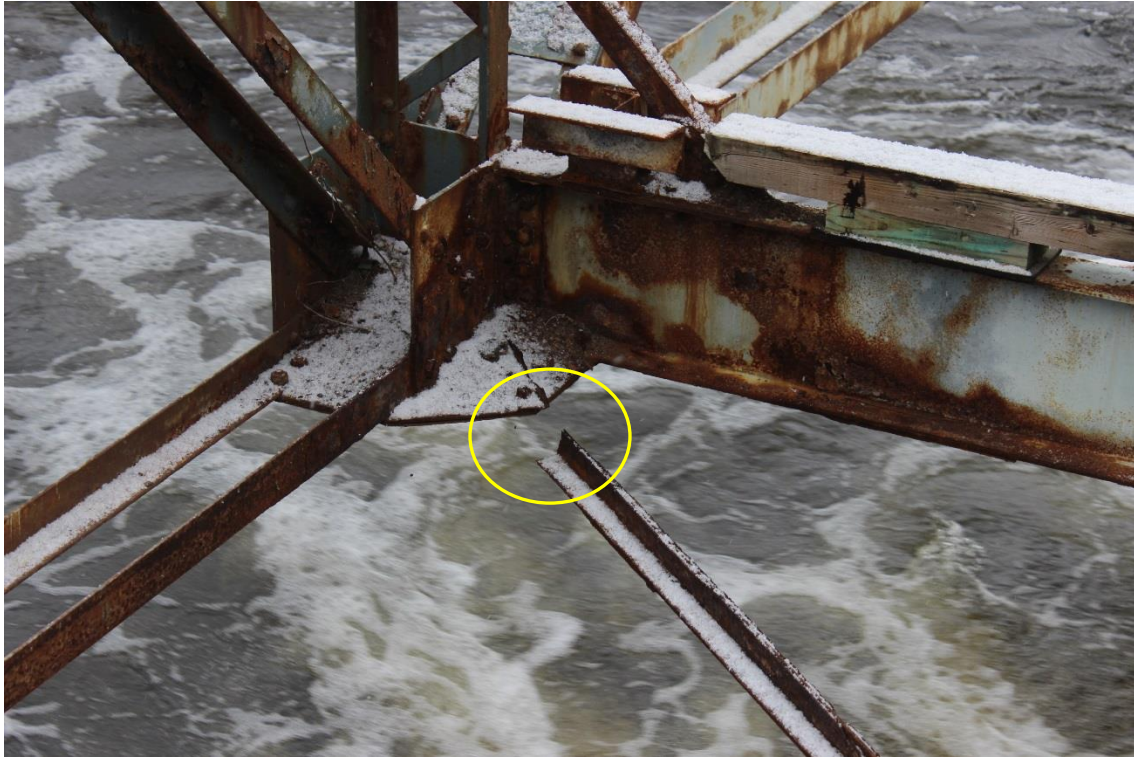
Image 3. West truss panel point 1 downstream severed diagonal brace
