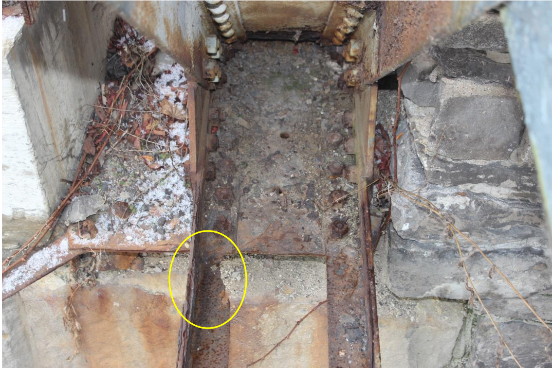
Image 7. Perforation, severe corrosion bottom chord east truss SE bearing area
