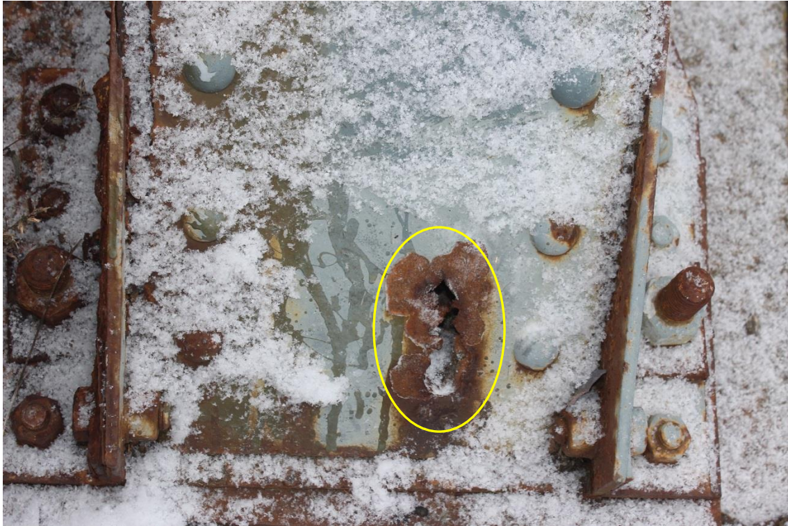
Image 11. Perforation of end diagonal cover plate NE bearing west truss
