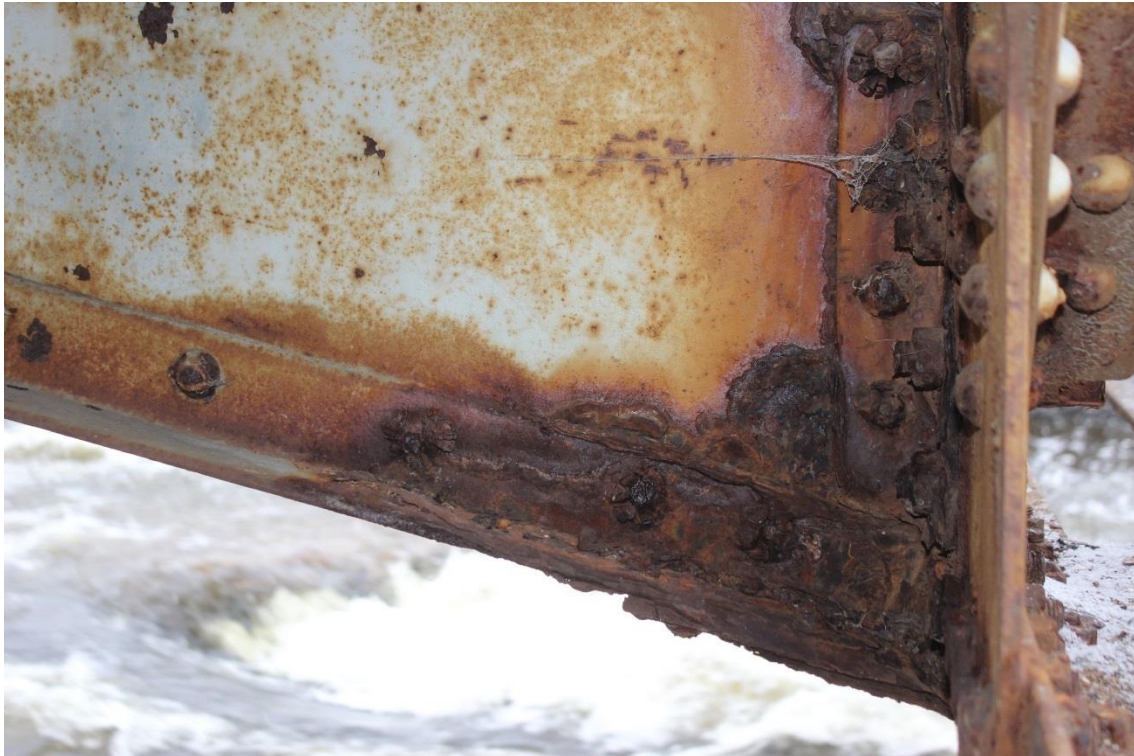
Image 8. Corrosion of sidewalk outrigger panel point 4 east truss
