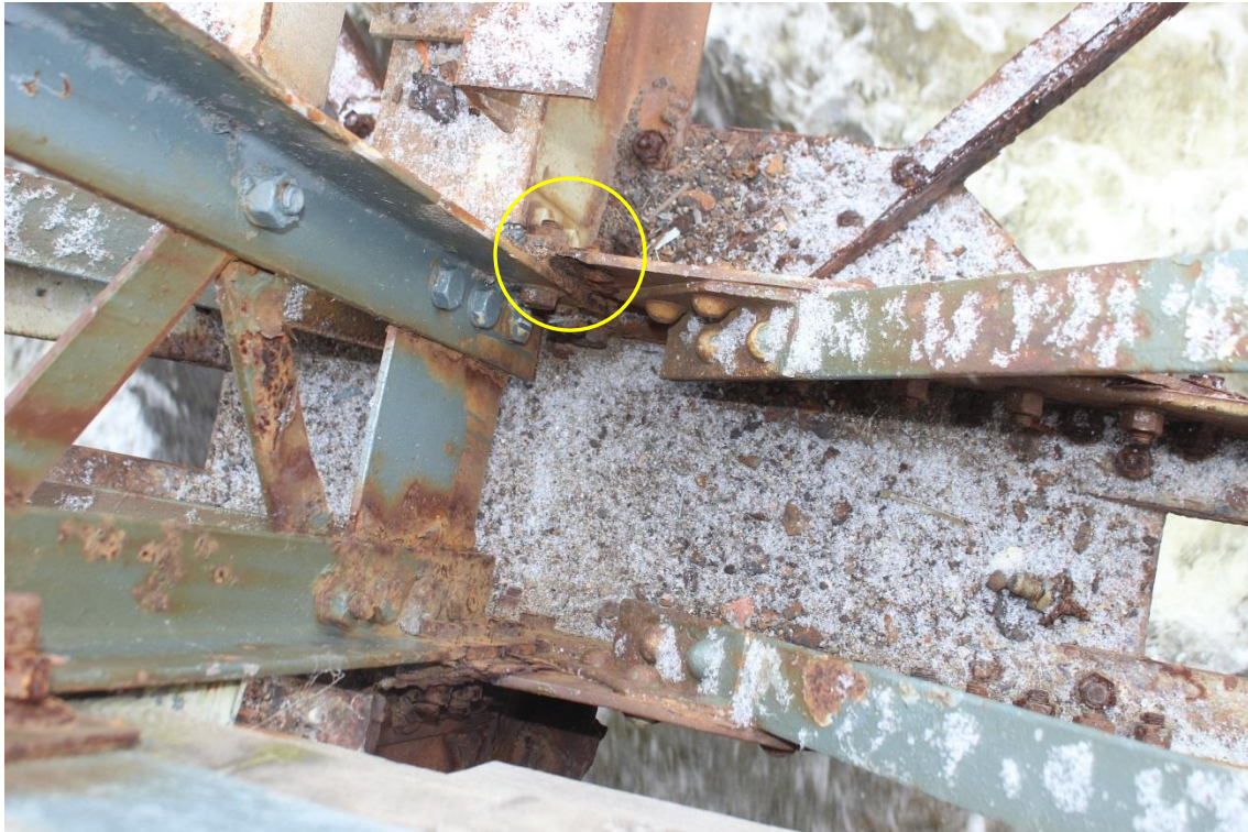
Image 10. Typical panel point east truss upstream side with gusset thinning
